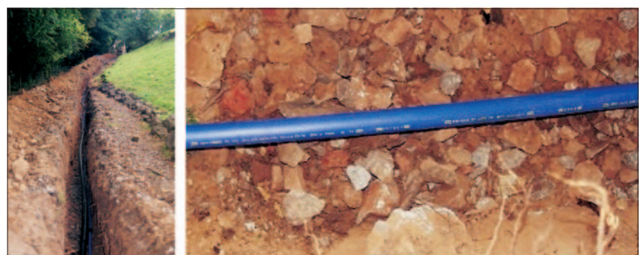
Fig. 8: Experimental installation (length 300 m) of polyethylene pipes without sand-embedding in rocky soil (limestone)
